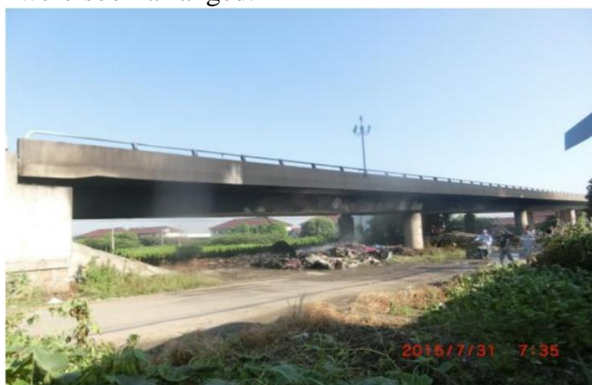
Fig. 4. Fire-damaged S12 bridge.
